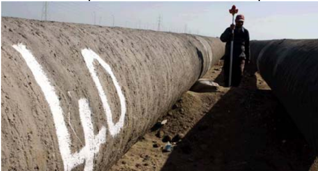
Gas pipeline in Egypt: “the objective is to maximize the volume of gas that can be transmitted in the pipeline every day”
